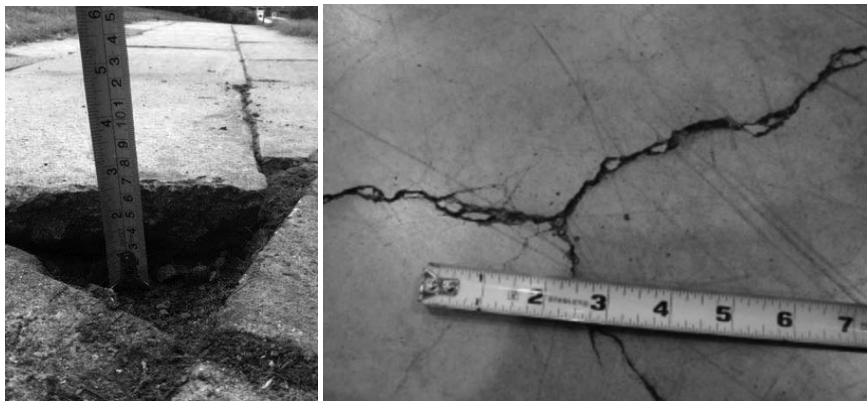
Figure 1: Measurement of pot holes and cracks of road
