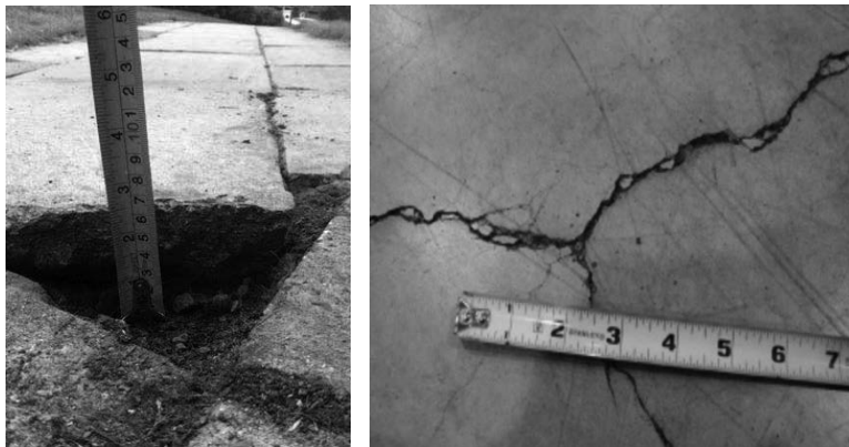
Figure 6: Measurement of pot holes and cracks of road
