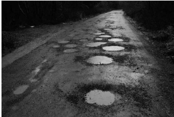
Figure 2: Formation of pot holes on Bituminous road surface.
