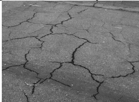
Figure 3: Formation of cracks on bituminous road surface.
