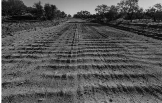
Figure 1: Corrugations on road surface
