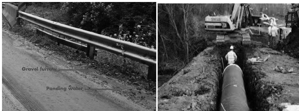
Figure 2: Improper Road side drainage and Provision of Drain Pipe
