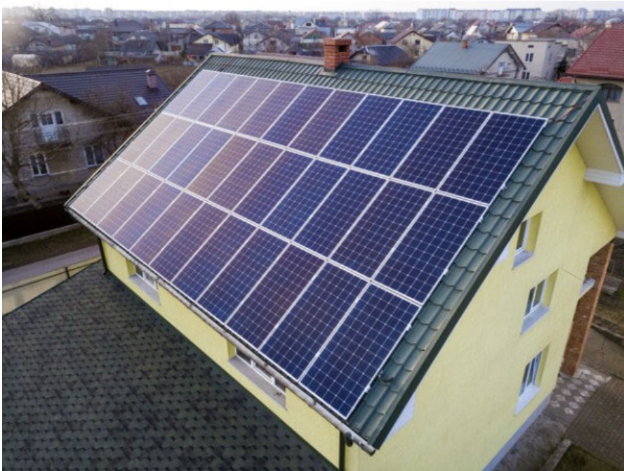
Fig. 2.19: Photograph of a roof top solar PV power system
