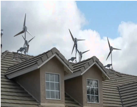
Fig. 4.15: Rooftop small wind turbine
