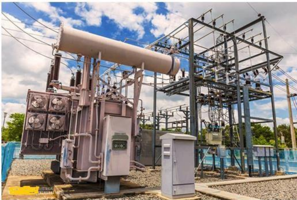
Fig10.1. Transmission line substation
